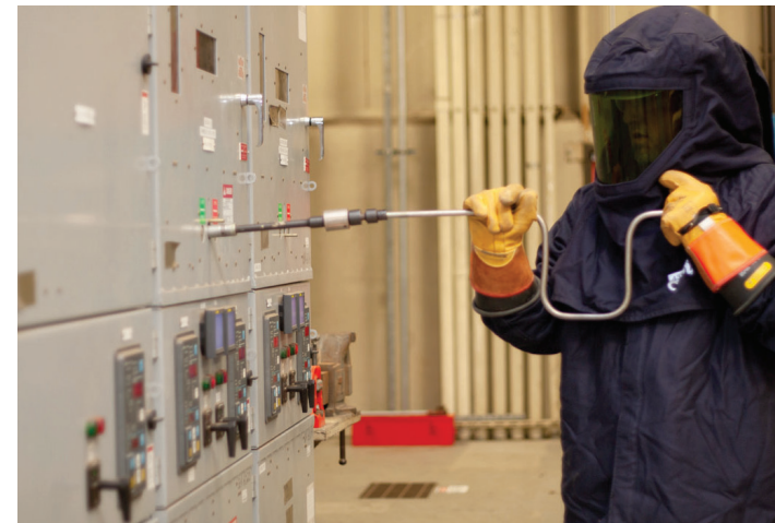
Building Automation and Control System sub-station maintenance at commercial customer's facility in Mossville, IL.
